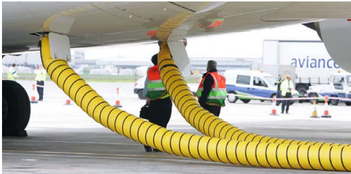
Yellow pipes making a big difference - these deliver pre-conditioned air to aircraft parked at Heathrow and airports all over the world.
